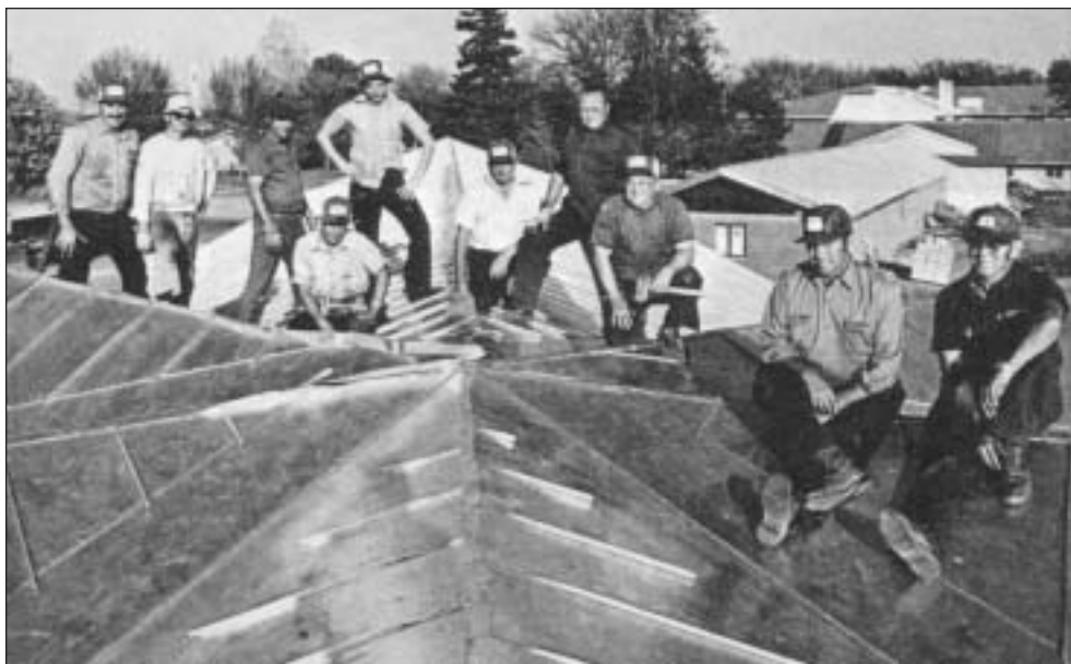
Roofing crew for the Hope Residence begun in 1975: (L-R) Pastor Bob Schlicht, David Hanke, Henry Koepp, Edwin Harms, Rick Carlson, Reno Carlson, Ewald Hauer, Pastor Paul Hanke, Reuben Tesch, and Paul Manthe.
